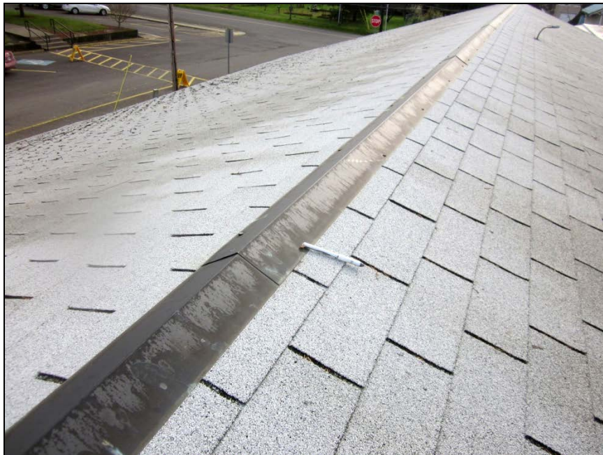
Sec. 1.02 – Roof A: View of typical fastener backing out at ridge cap at center section of the roof.
