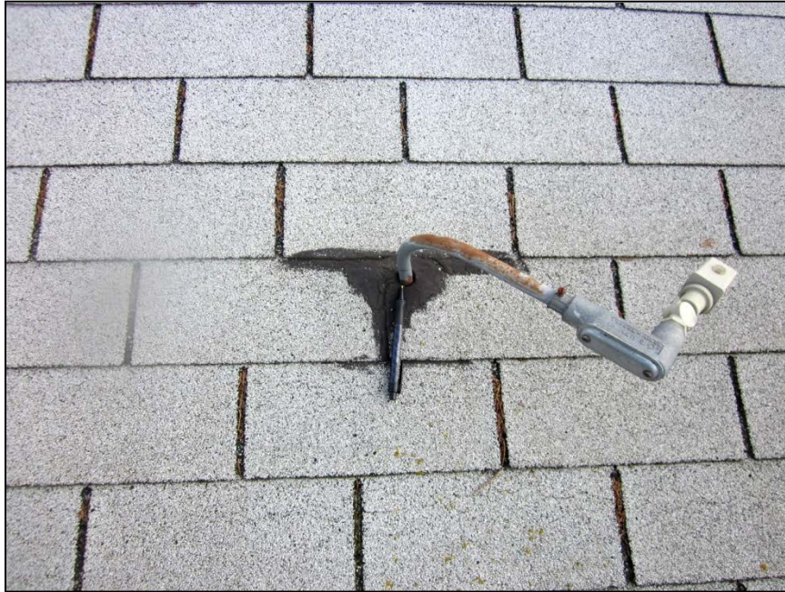
Sec. 1.03 – Roof A: View of void in mastic at pipe penetration near ridge line at south section of the roof.
