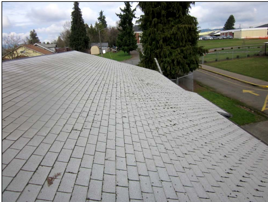
Sec. 1.04 – Roof A: View to north of moss growing at northeast section of the roof.
